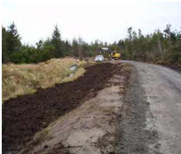
Photo 4: Example of excavate and replacement access track verge reinstatement with peat turves
