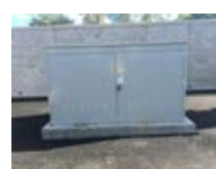
INDICATIVE PRIMARY METERING CABINET
