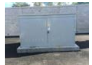
INDICATIVE PRIMARY METERING CABINET
