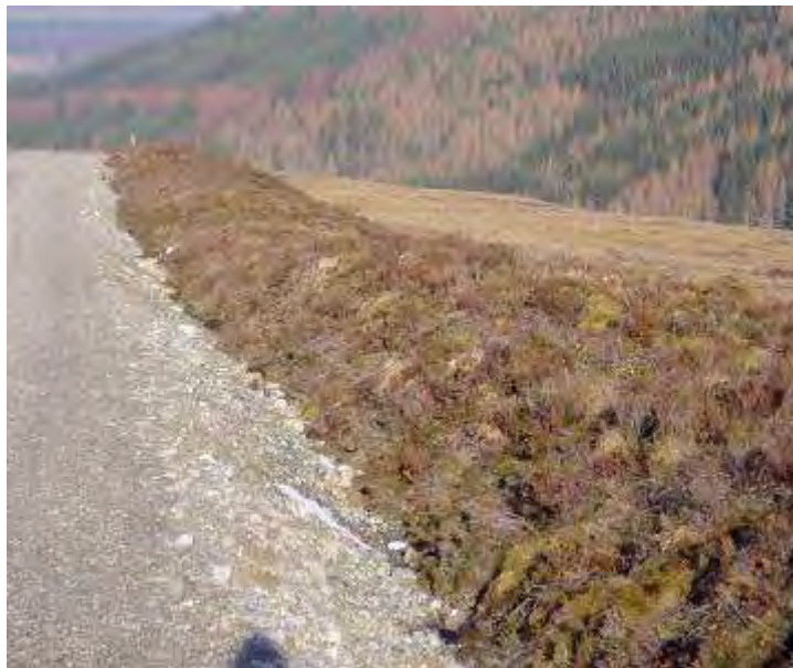
Photo 3: Example of good track reinstatement with heather turves re-established
